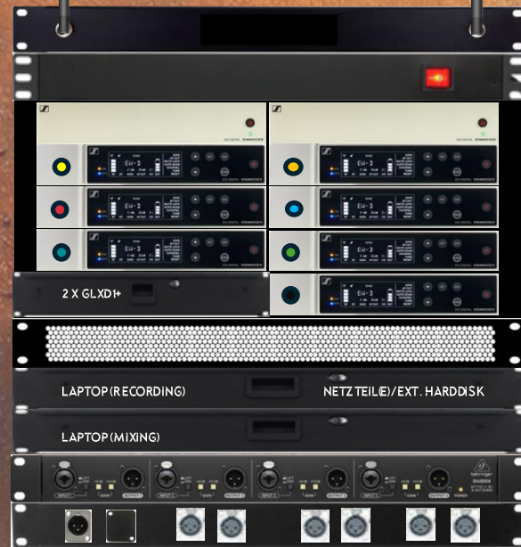
STAGE RACK (LEFT)
