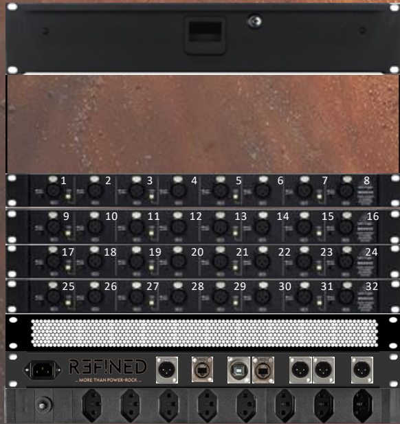
MAIN RACK (REAR)
