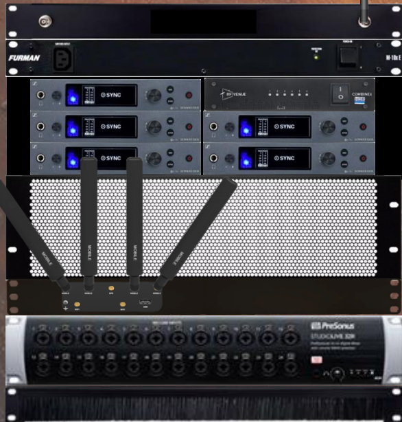
MAIN RACK (FRONT)
